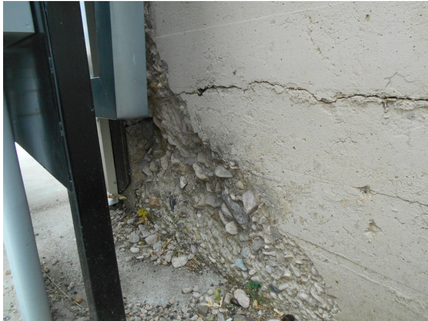
Photo 3: Damaged section of concrete wall on north east side
