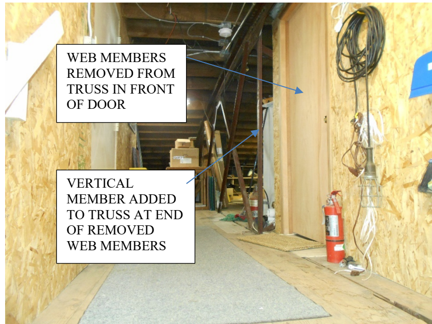
Photo 4: truss with web members removed
